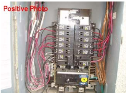
Photo: 5. View inside of electric panel. (1)
